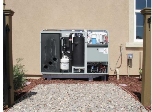
This is what the water recycling system looks like with the cover taken off. It also includes an in-ground storage tank that can hold 250 gallons.
